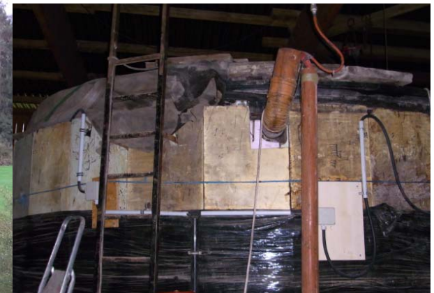
Biogas generation plant
